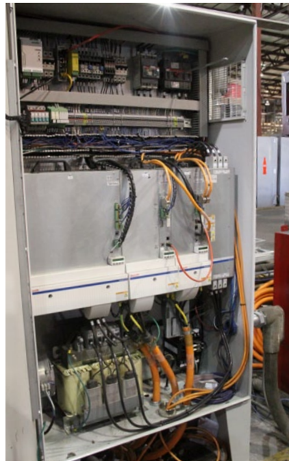
Antiquated analog controls and motors were replaced with IndraDrive M servo drives and asynchronous motors that return wasted energy to the system.
