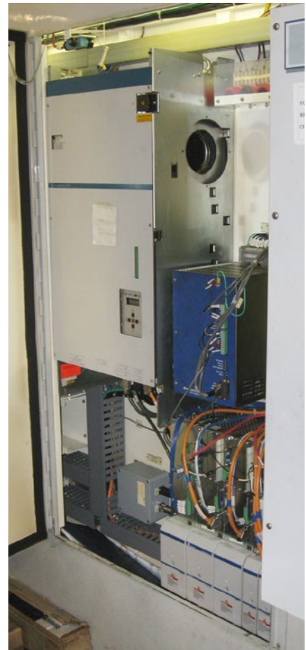
New Rexroth drives help extend the operational life of four contour grinding machines at Cummins.
