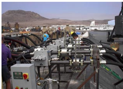
With the rocky coastline of Baja, Calif., as a backdrop, the main hydraulic valve stand features four Rexroth custom high-flow manifolds and six Rexroth 4WRZ25 proportional valves.
