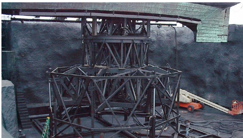
Hydraulic Controls Inc. provided the hydraulic components to power a gimbal (multi-axis motion platform), which controlled a full-size replica of a 19th century naval frigate. The gimbal measured 40 feet tall with a 40-foot base and weighed 60 tons.
